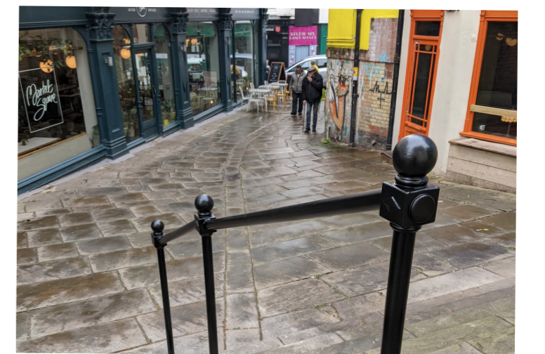
Repointing of the pavement and new handrails installed off Rendezvous Street, Folkestone as part of public realm improvements funded by the 'Welcome Back Fund' during the year.
